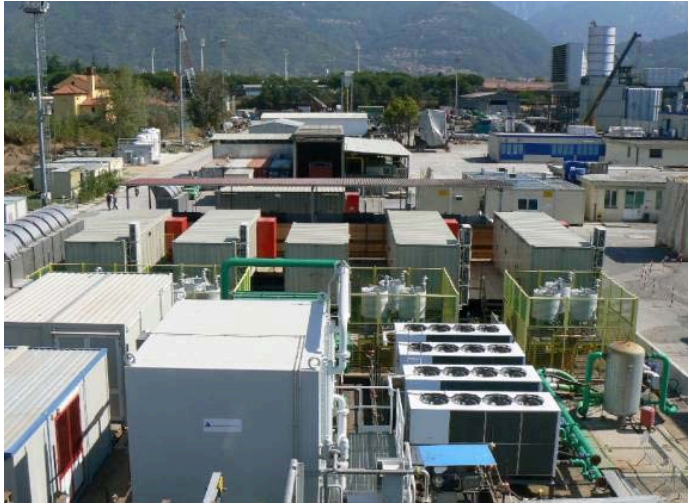
Figure 12: Drive system comprising the converters, inductors and the synchronous machine
